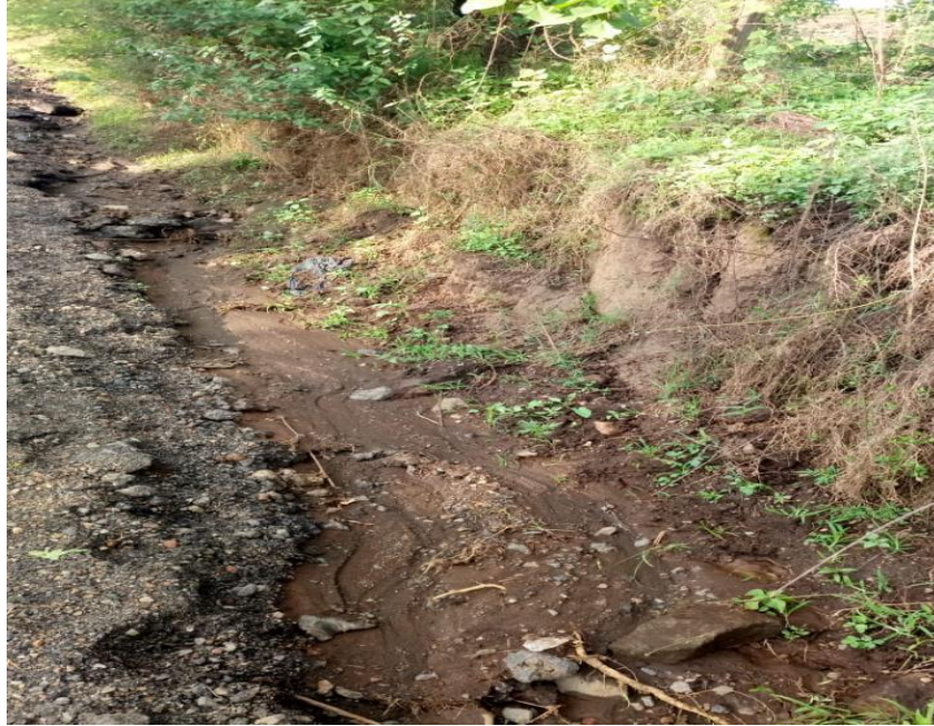
Plate 6.7: Current road to the project site being undermined by poor drainage
