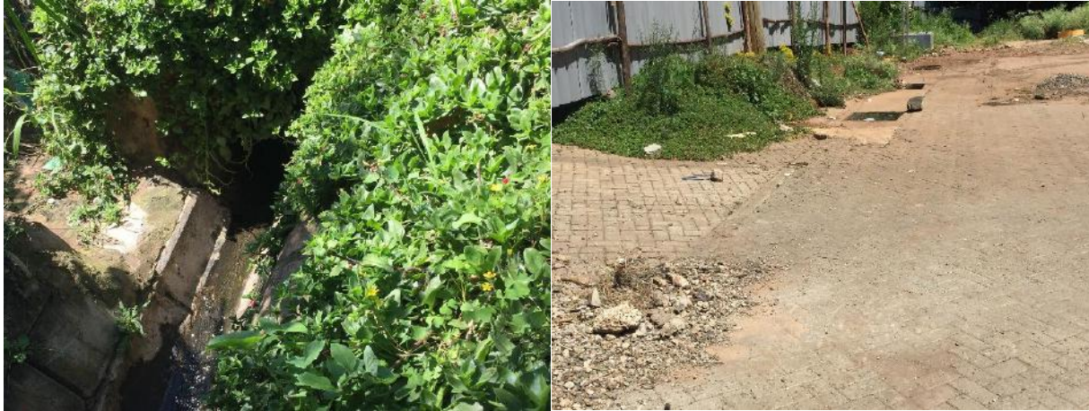
Photo 12 & 13: NCWSC's storm water drainage system at the project site
