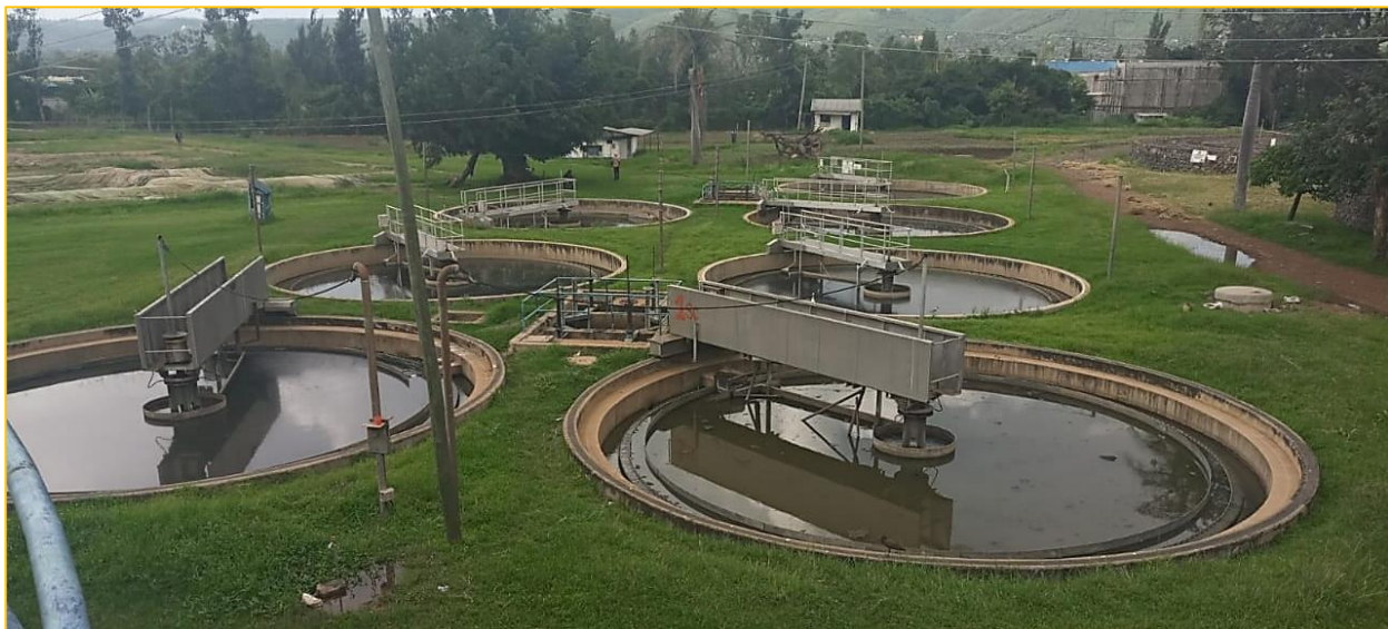
Figure 41. A section of the Kisat Sewage Treatment Plant showing the settlement tanks (Source: Site visit, November 2019).
