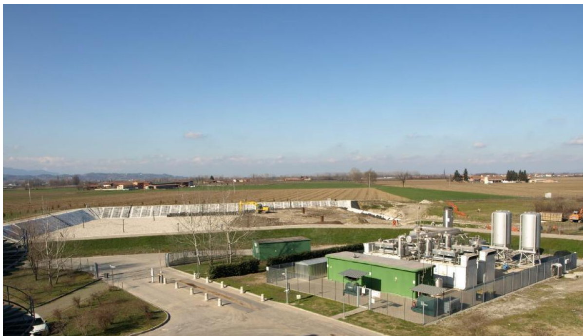
Plate 1 ISWM Plant - Bioreactor and a biogas treatment and energy recovery system
