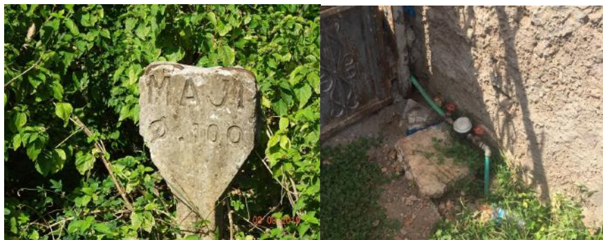
Figure 7 Pipe water infrastructure at Msumarini &amp; metered connection to project site
