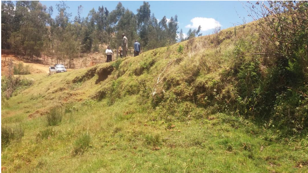
Figure 38 The old wall of the ExJacob Dam. The wall is in bad shape and is leaking
