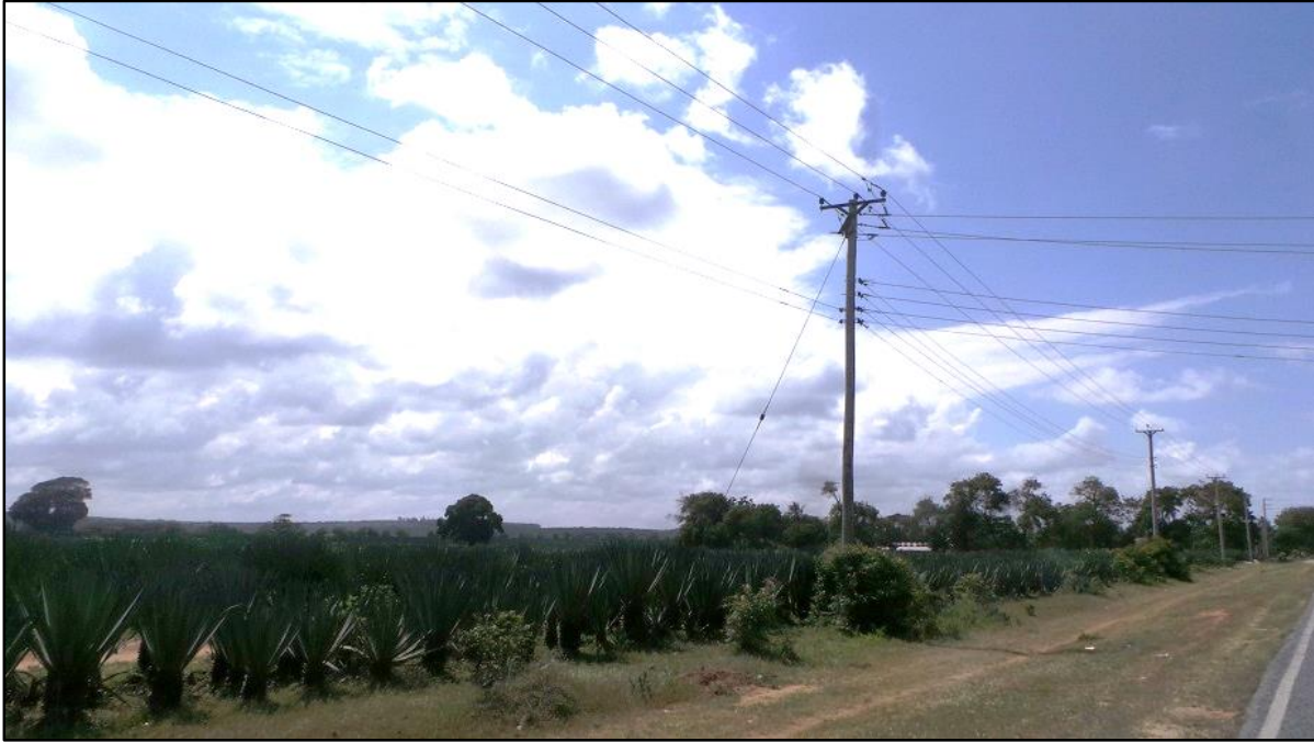
Plate 14: Power lines in Vipingo Area
