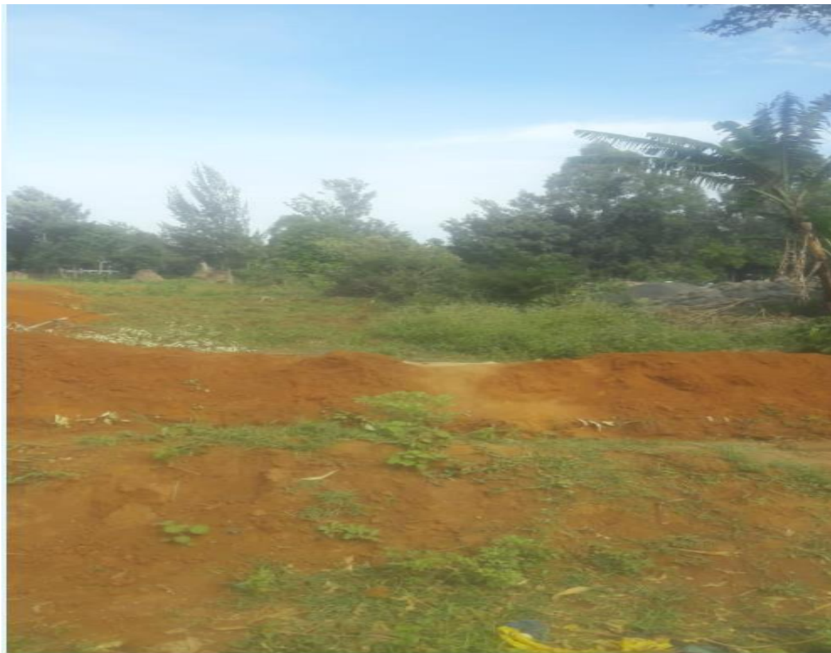
Figure 1: Part of the plot to be developed for LPG Storage and Filling Plant with the construction of the perimeter wall ongoing.
