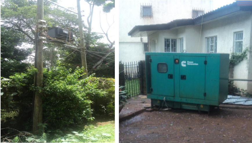
Plate 12: Electricity Transformer and Generator
