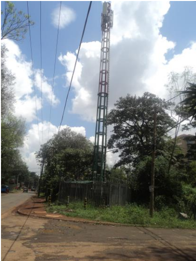
Plate 13: Communication Booster along Riverside Drive
