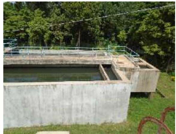
Stilling Well and 2 Nr. Sedimentation Tanks capacity 3,500m 3 /d at Kiang'onde Treatment Works.
