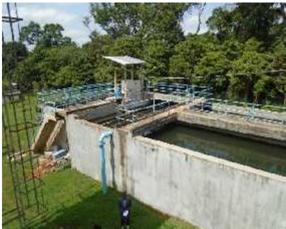
Sedimentation Tank, Filters and Chlorination units at Kiang'onde Treatment Works.
