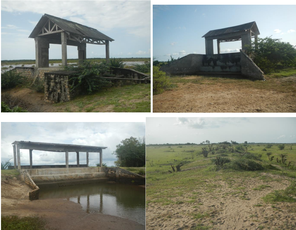
Plate 1: Remnants of pump station 3, 2 & 1 and one of the disintegrating dykes on site
