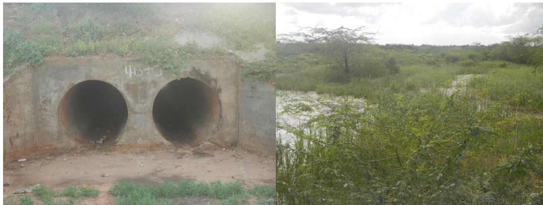
Plate 5: A section of Kwa Kubanda stream note that water was available downstream after the culvert
