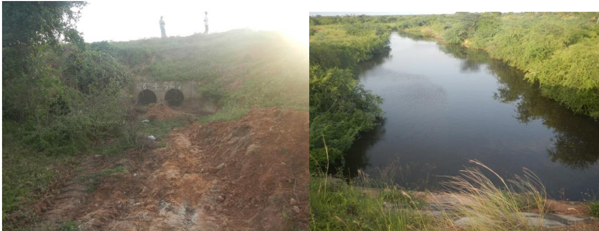
Plate 4: A section of the Mbwageni stream note water was downstream past the culvert at the road
