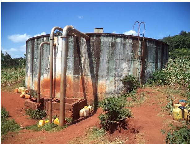
Figure 2-7 The existing Iveti tank to receive additional supplies of water
