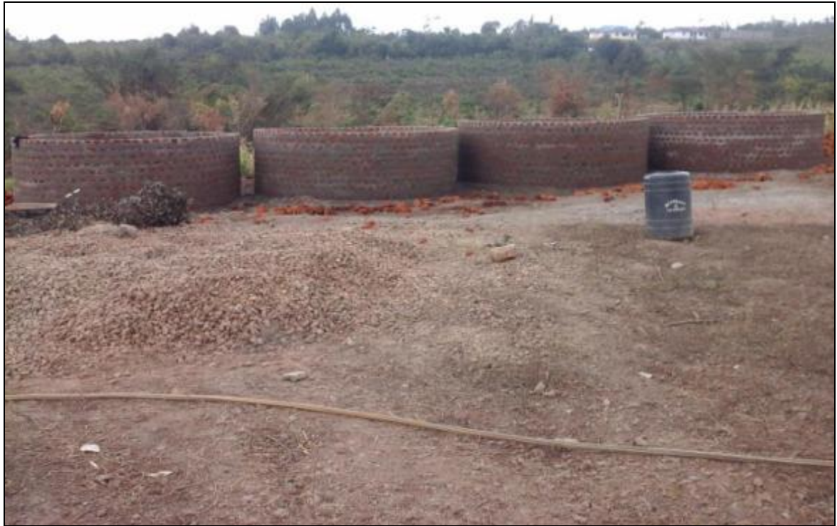
Plate 1: The Leaching Tanks
