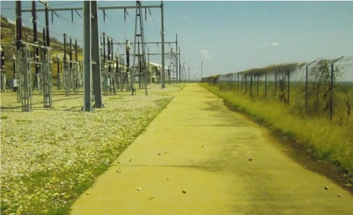
Substation at Turkwel
