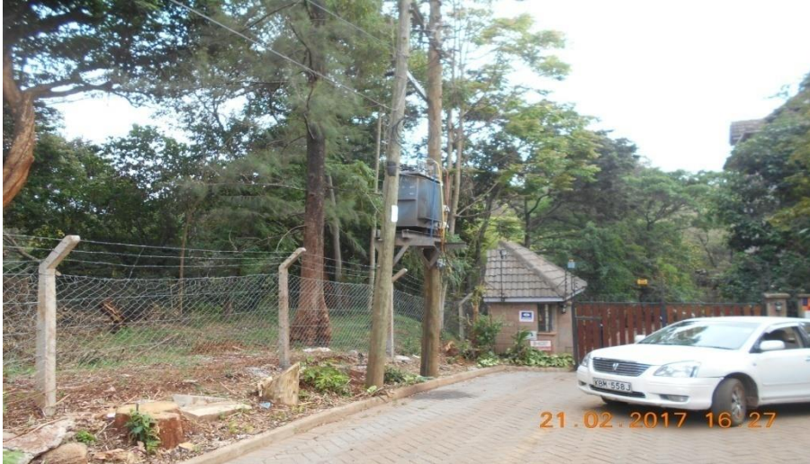
Figure 3: Electricity transformer situated about 30 m for the main gate of the site. Source Field Work, 2017.
