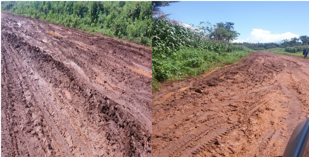
Plate 6: Current state of the Main Kitale-Endebess-Suam road that stands to be improved should the border town at Suam be established
