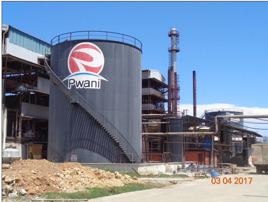
Figure 4: A section of the existing installations at the facility
