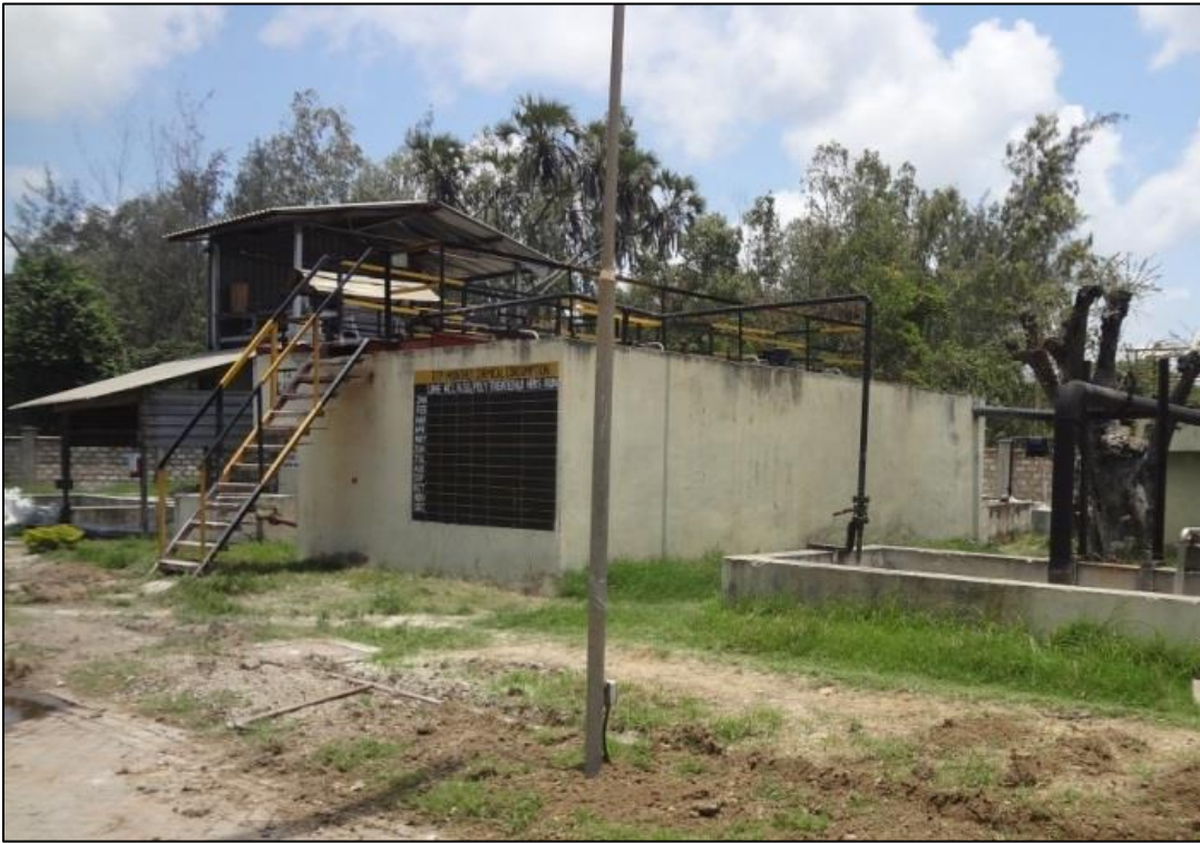
Figure 6: Waste water treatment plant installed at the facility
