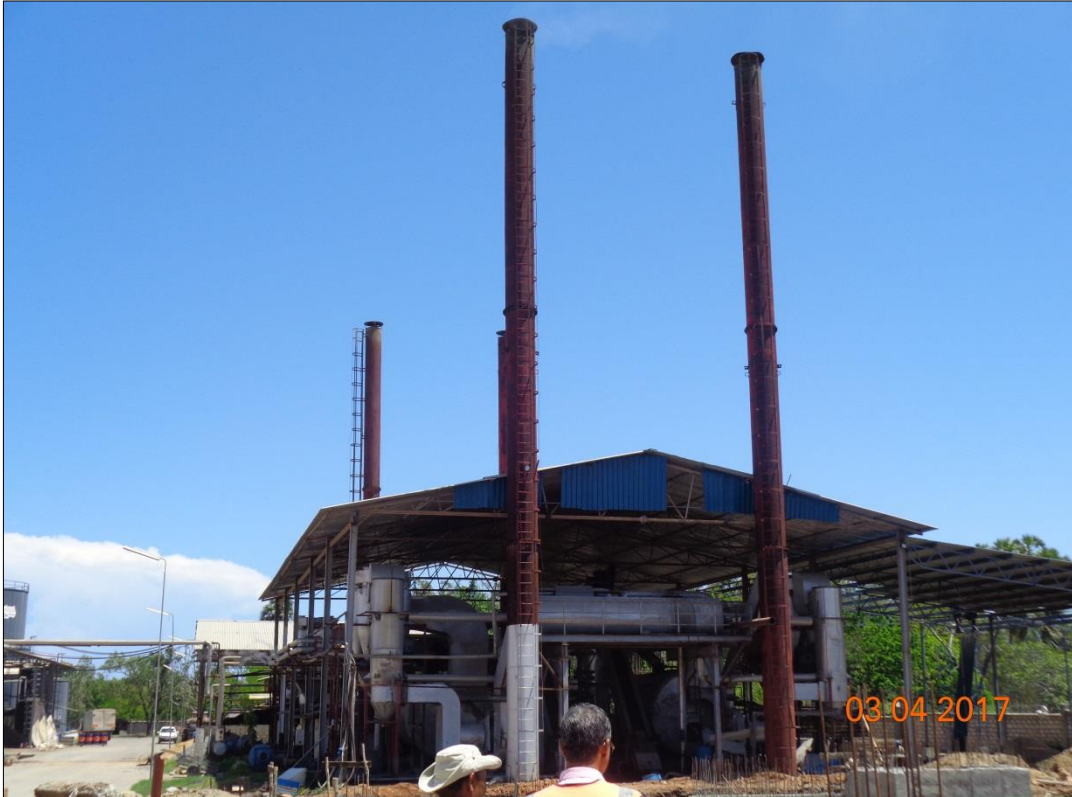
Figure 5: Showing the existing boilers and cooling towers installed at the facility
