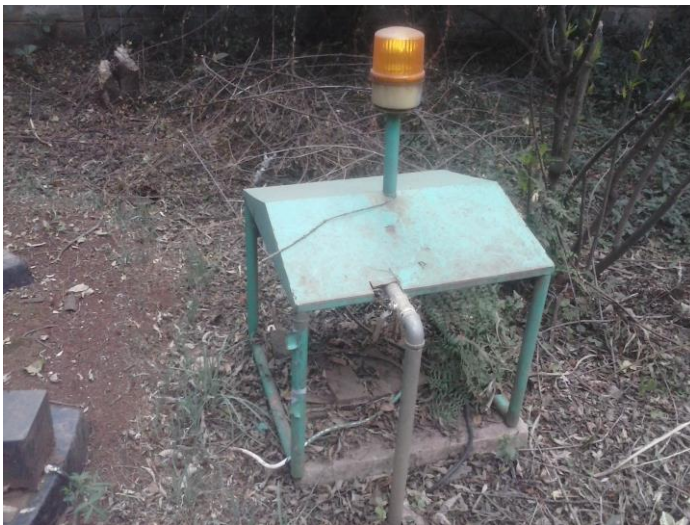
Plate 4: Water meter and water tank
