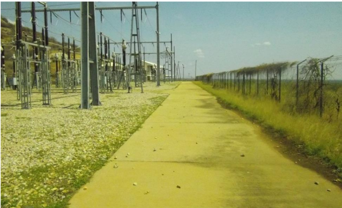
Substation at Turkwel
