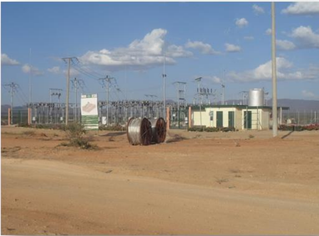
Rural Electrification Authority Substation (36N, 0776631, 0235122) located by the road side. It is 900m from the TL
