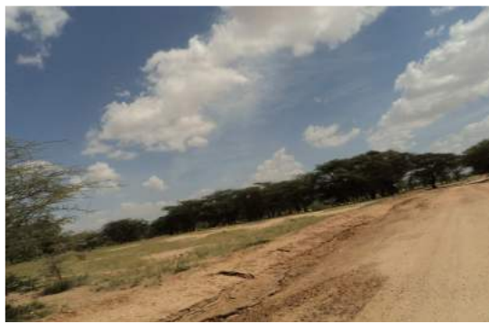
Plate 3.2(c): Scoured section on the existing road alignment
