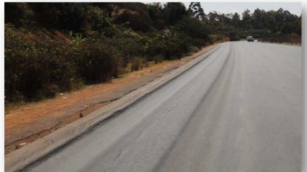
Rutting on the left lane used by heavy vehicles
