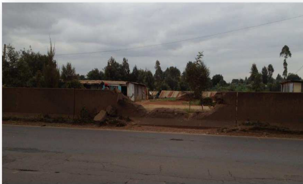
Damaged New Jersey barriers which allow illegal crossing by pedestrians
