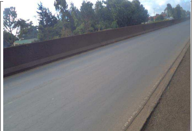
A Section of A104 with new jersey barrier that hinders unrestricted crossing by residents who opt to jump over it as opposed to using the available foot bridge, the residents propose that more crossing points should be established
