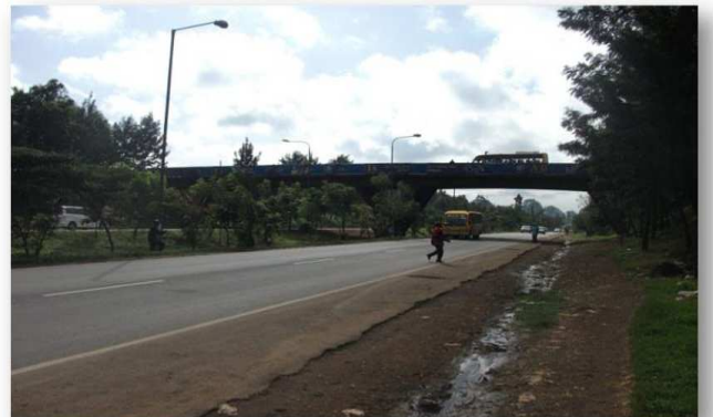
Project road lack of proper drainage
