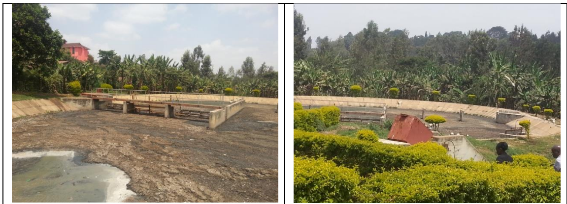
Figure 2: Existing Waste Water Treatment Facility.
