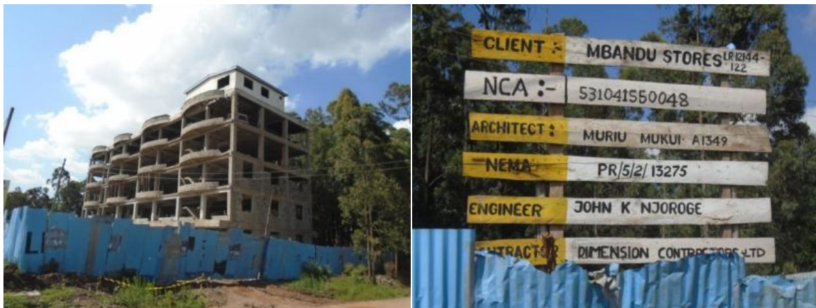
Plate 7: The five storey building under construction along Langata road within Karengata area
