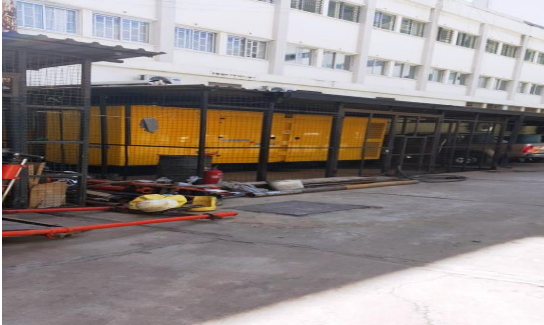
Picture 2: The backup generator on site
