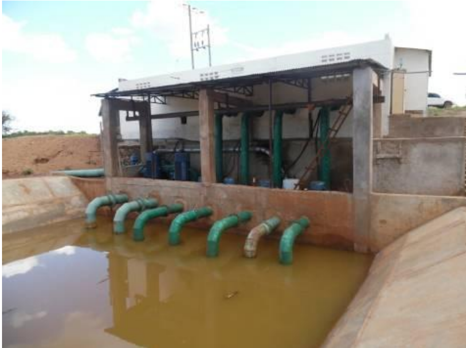
Plate 2: Irrigation infrastructure at Wikithuki Irrigation project, Kitui County
